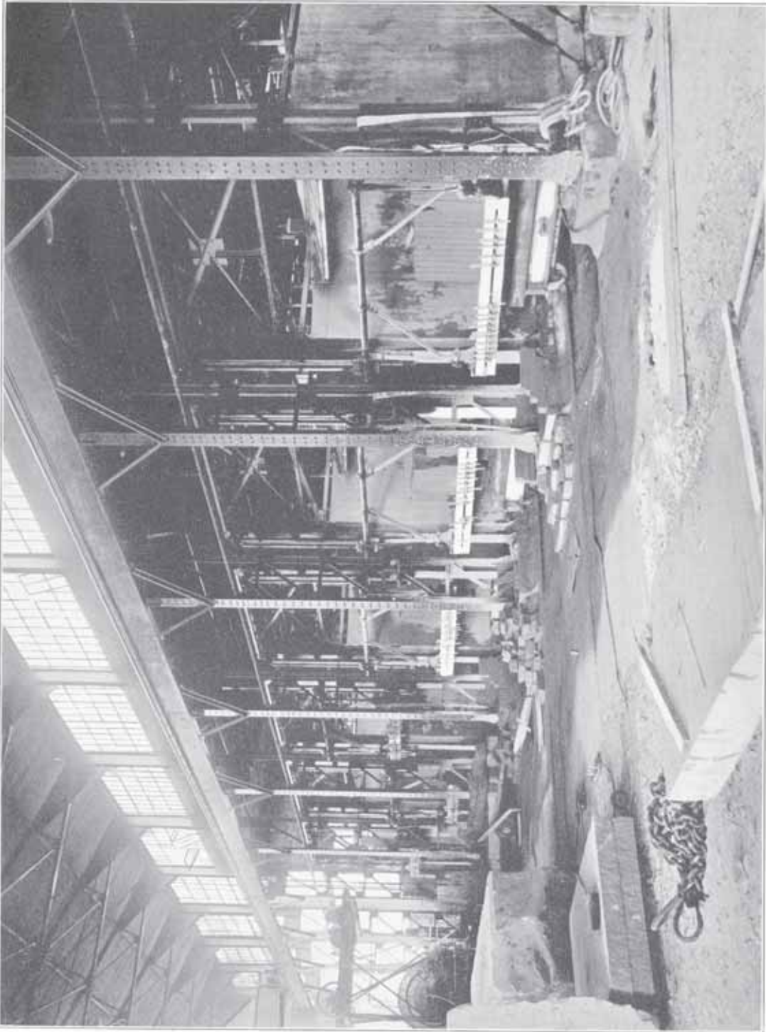
Installation of Six Bedford All Steel Gang Saws, Consolidated Stone Company, Bedford, Indiana
